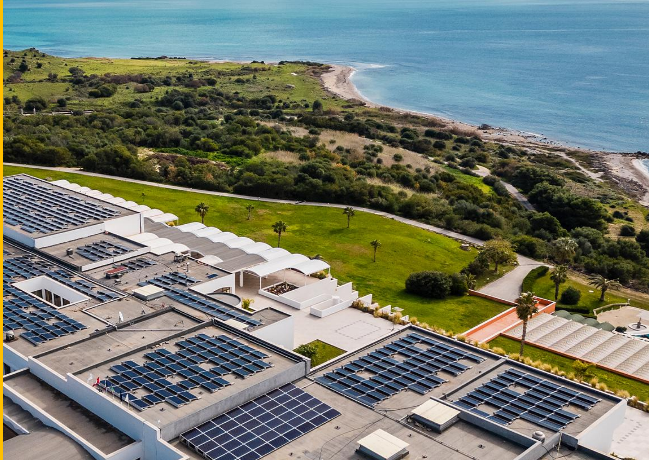
Sciacca (AG) - 312 kWp SunPower photovoltaic system
