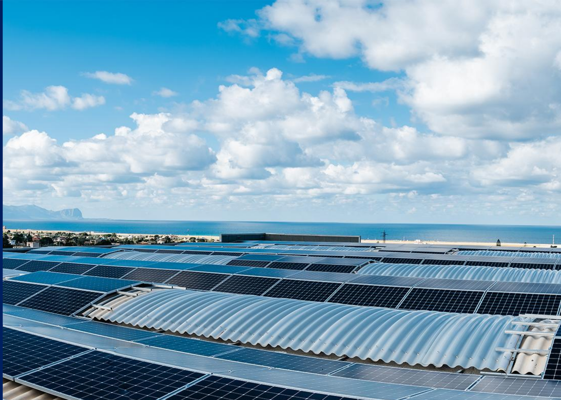
Cinisi (PA) – 616 kWp SunPower photovoltaic system
